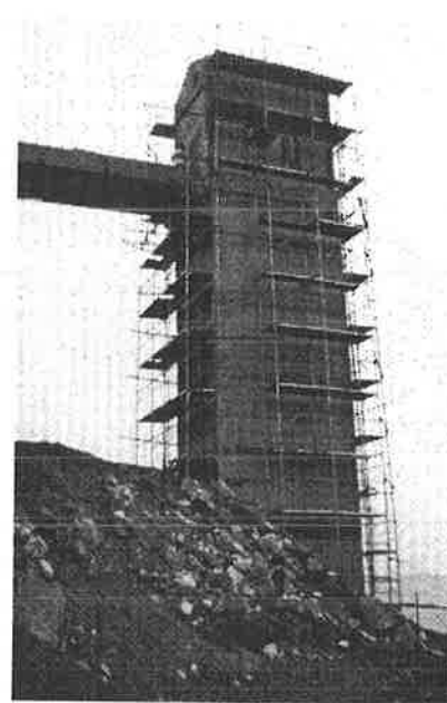
Water Tower in Mozambique That Was Partially Funded as Child Survival
